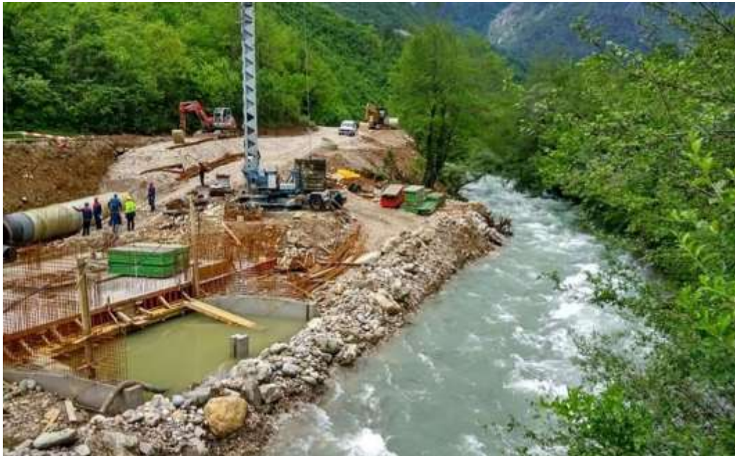
Small hydropower plant “Zlate”, river Doljanka, Jablanica, Bosnia and Herzegovina Source: https://zurnal.info/clanak/unatoc-presudama-ministarstva-nezakonito-odobravaju-gradnju-malih-hidroelektrana/24226
