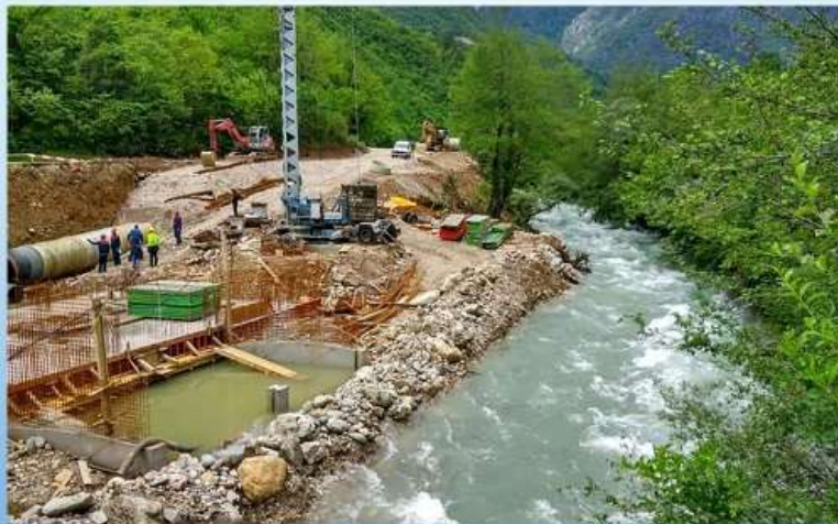
Photo 4. Small hydropower plant „Zlate“, river Doljanka, Jablanica, Bosnia and Herzegovina Source: https://zurnal.info/clanak/unatoc-presudama-ministarstva-vezikonita-odolazivo-gradnja-iz-salt-hidroelektrana/24226
